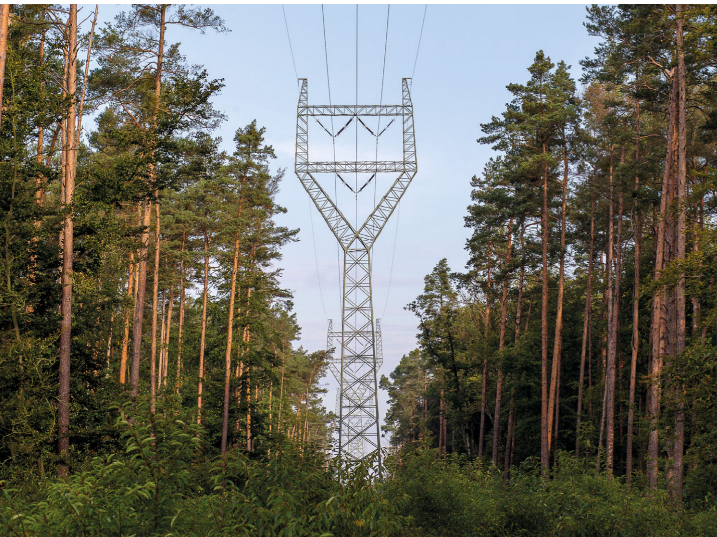
PSE, Linia 220 kV Glinki – Reclaw
